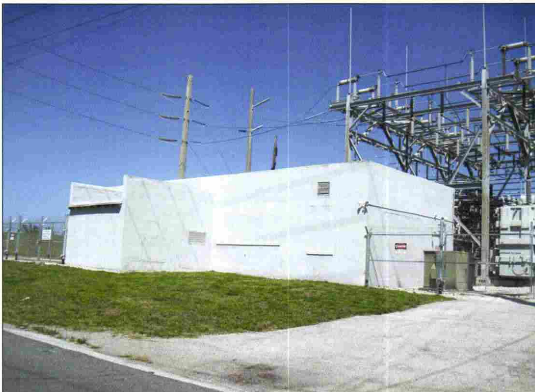
Photograph 2. View of substation, facing northeast (PCI March 2010).
